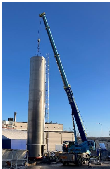
Silo i Aluminium, 1st, 120m 3
